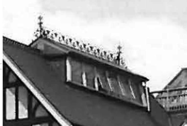
Original photograph detailing roof top lantern and roof finials to the Original Beecroft Gallery
