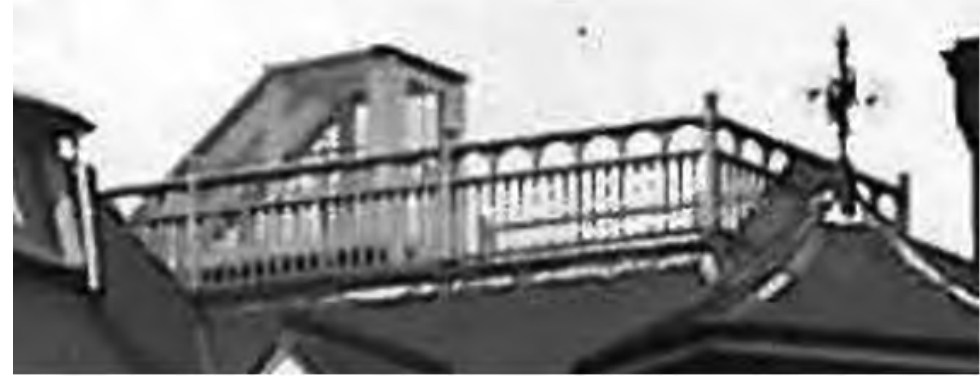
Original photograph detailing roof top access, feature balustrade and handrail, roof finial and roof top lantern to the Original Beecroft Gallery
